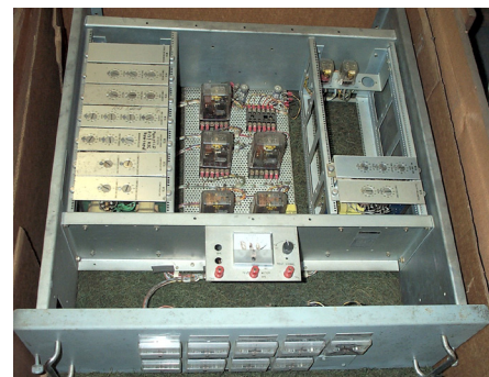
Figure 3: WTA Regulator Logic Module are replaced
