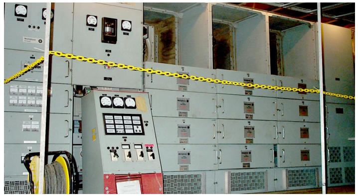
Figure 1: WTA voltage regulator/exciter
