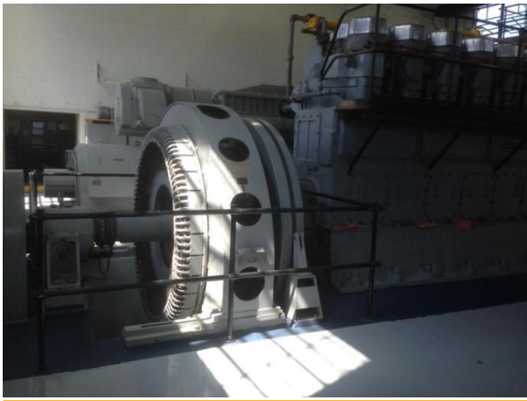
Figure 3. Horizontal Generator with Belt Driven Exciter
