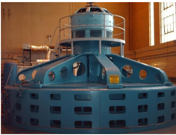
Figure 2. Salient-Pole, Vertical-Shaft Hydro Machine
