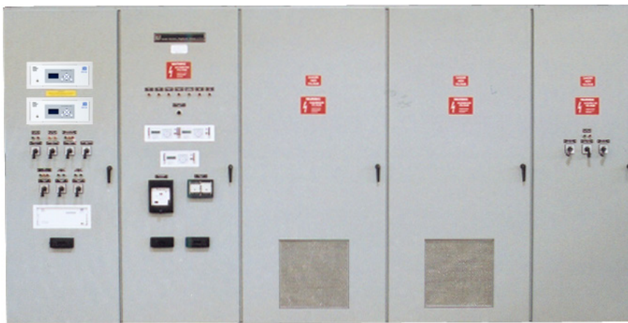
Figure 2: Dual DECS-450/dual 2500 Amp bridge system.
