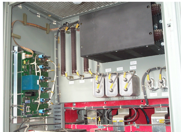
Figure 6: Gate pulse amplifier boards are also targeted for removal.
