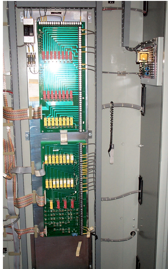
Figure 5: Input/output boards are removed.
