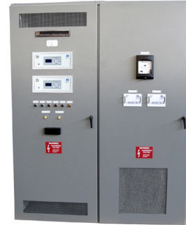
DECS-450 Cubicle - dual voltage regulator exciter
