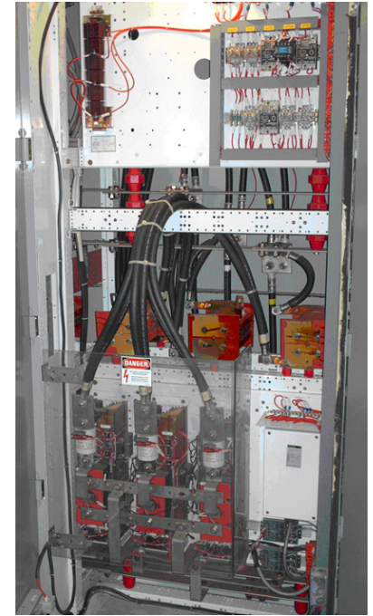
Figure 2: Retained Bridge Rectifier and current sharing reactor
