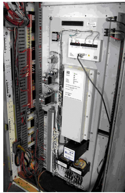
Figure 5: New subpanel to replace original MGR modules
