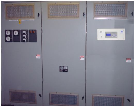
Figure 10: Two Bridge MGR Excitation System Updated with DECS-450 for Digital Control
