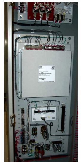
Figure 8: Basler Firing Circuit Chassis for Westinghouse Powertrex /PRX Voltage Regulator Retrofit
