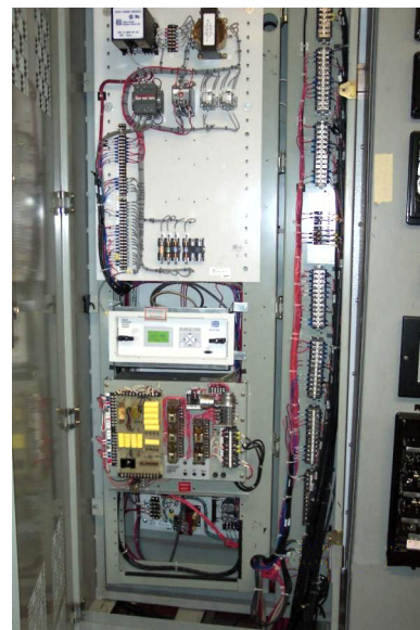
Figure 7: DECS-400 Replacement of PRX 302 Voltage Regulator on Westinghouse 501 Generator
