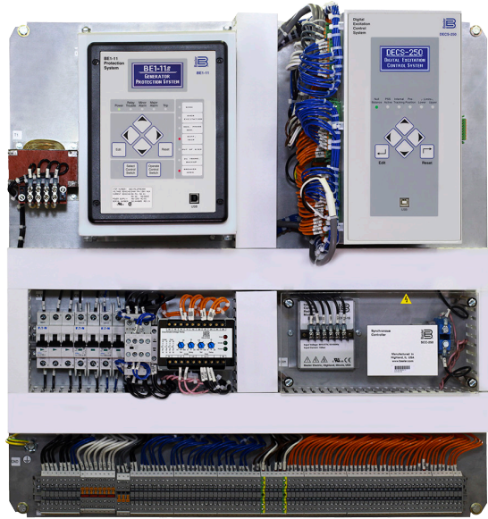
Figure 7: Prepackaged Basler SGC-250 systems replace exciter field rheostat and voltage regulator
