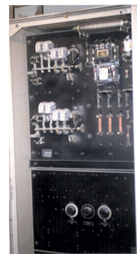
Figure 4: A system with field switches and an Amplidyne voltage regulator
